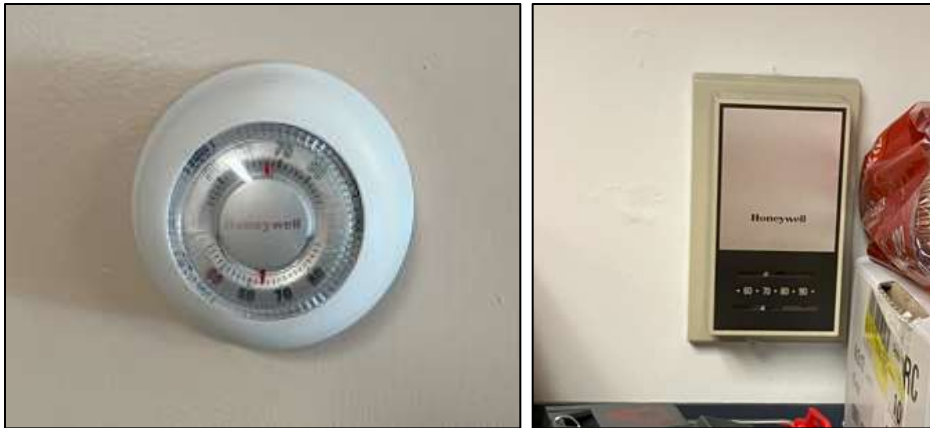
Existing thermostats in office and food pantry
